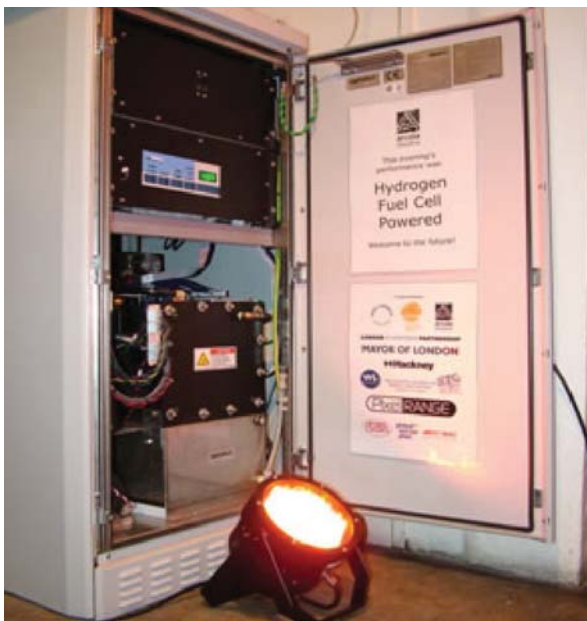
Arcola's hydrogen fuel cell
