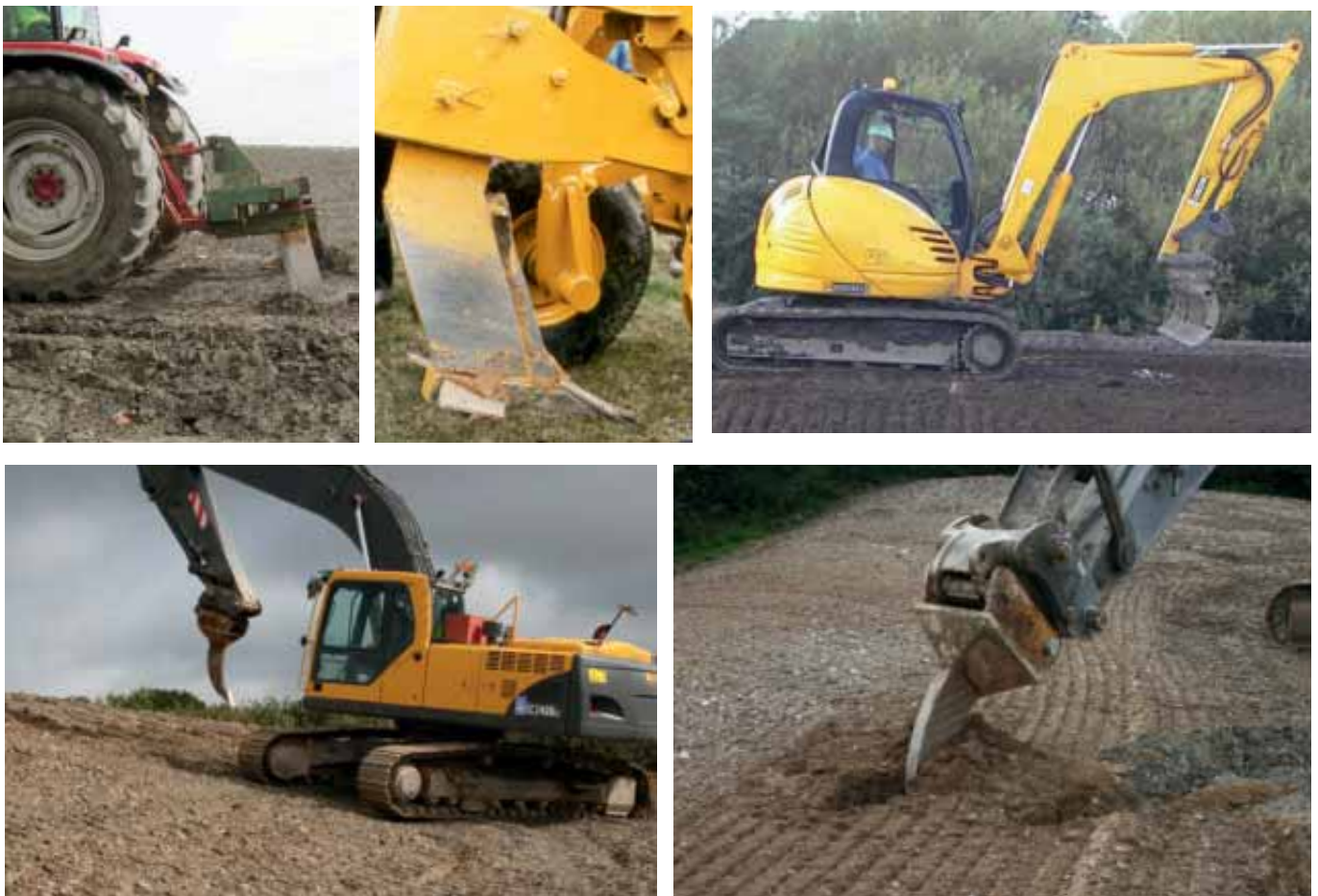
Top (from left to right): Ripping by tractor-drawn tines, Large winged-tine ripper, Topsoil rake used on a 3 tonne excavator
