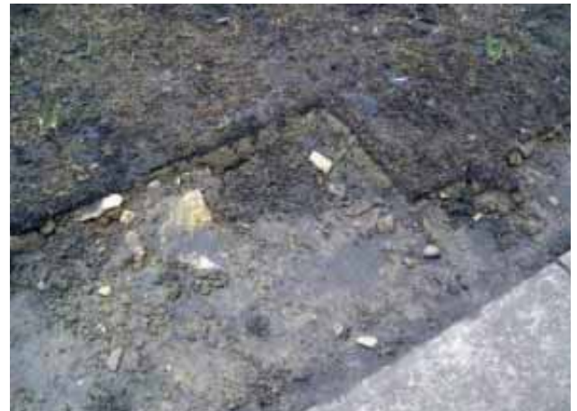
Surface water running onto adjacent paving
