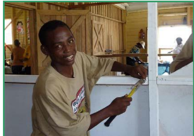
A trainee carpenter helps refurbish the All Saints community centre in New Amsterdam, Guyana, along with other women workers as part of a vocational training course funded by DFID through UNDP's Enhancing Public Trust, Security and Inclusion programme
