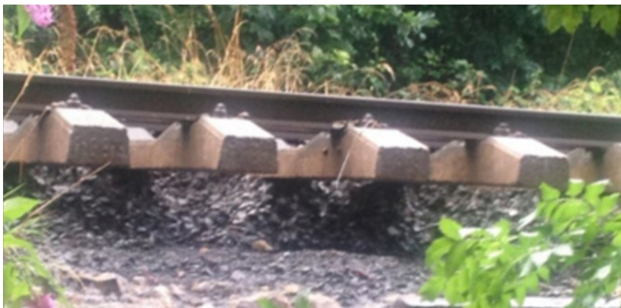
Figure 13: The unsupported track section following the washout in 2012
