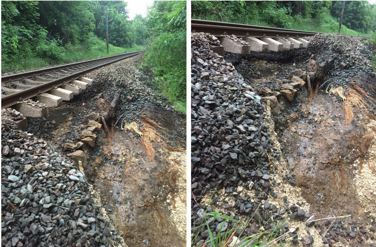
Figure 2: The washed out track and the embankment
