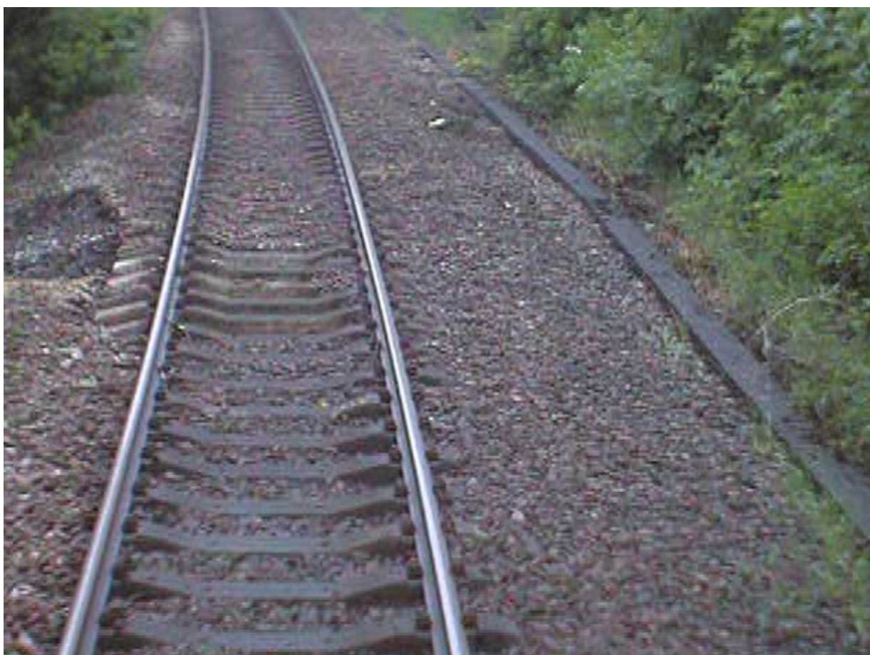
Figure 8: Still image of the track damage taken from the forward facing CCTV footage from train 2D73 (image courtesy of Northern Rail)
