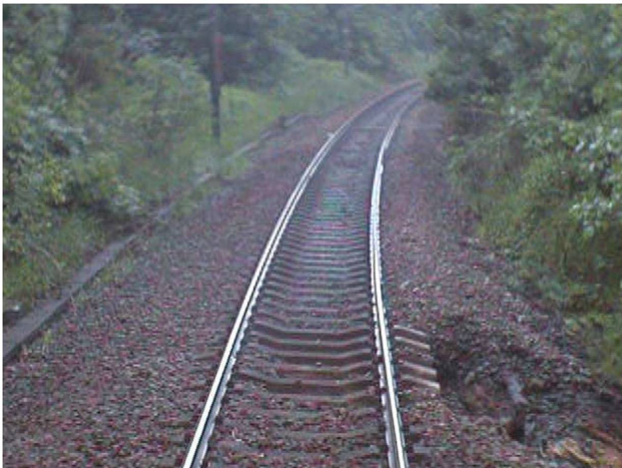
Figure 7: Still image of the track damage taken from the forward facing CCTV footage from train 2D72 (image courtesy of Northern Rail)
