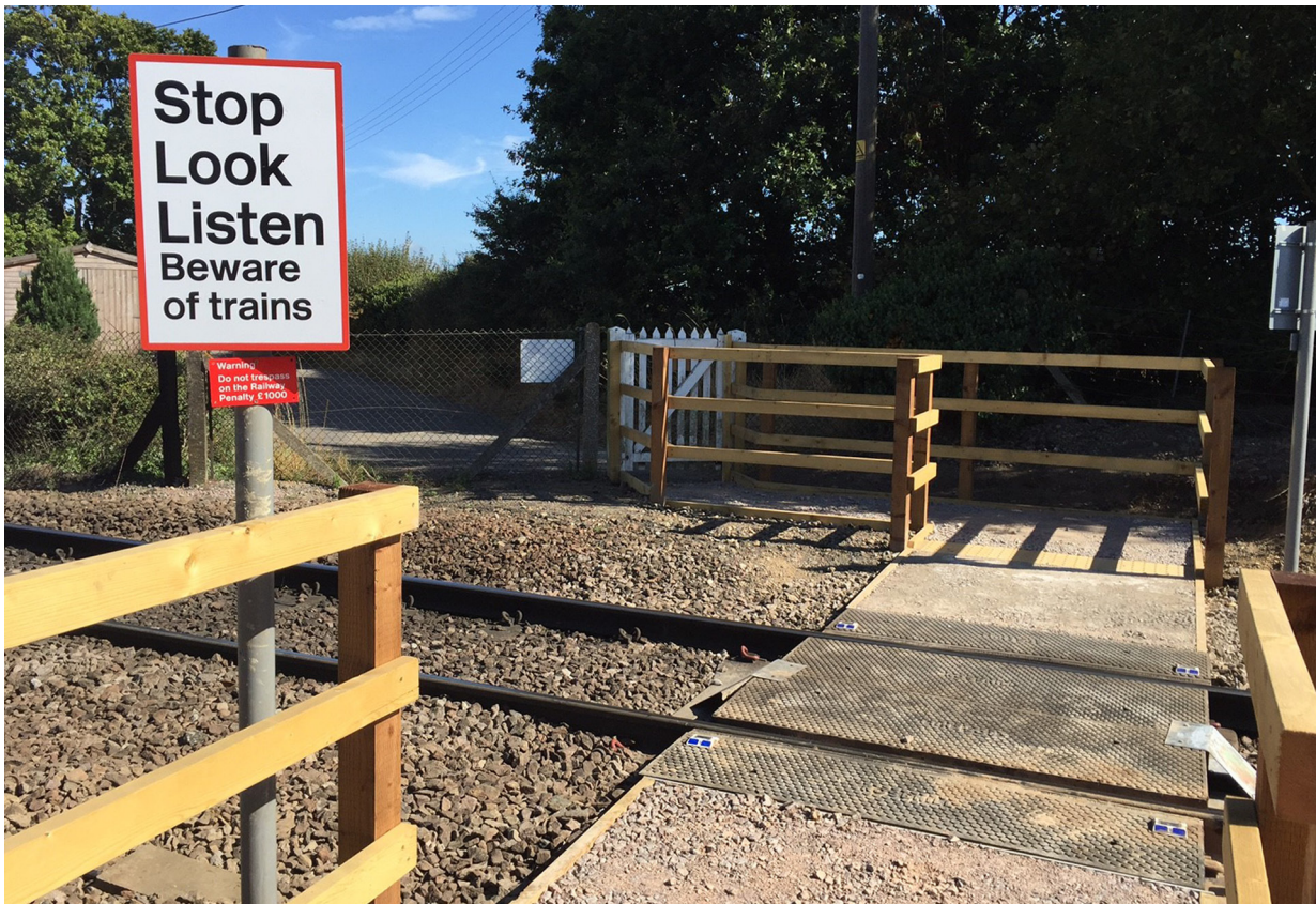
Figure 13: New crossing deck and fenced approach paths at Grimston Lane footpath crossing (image courtesy of Network Rail)
