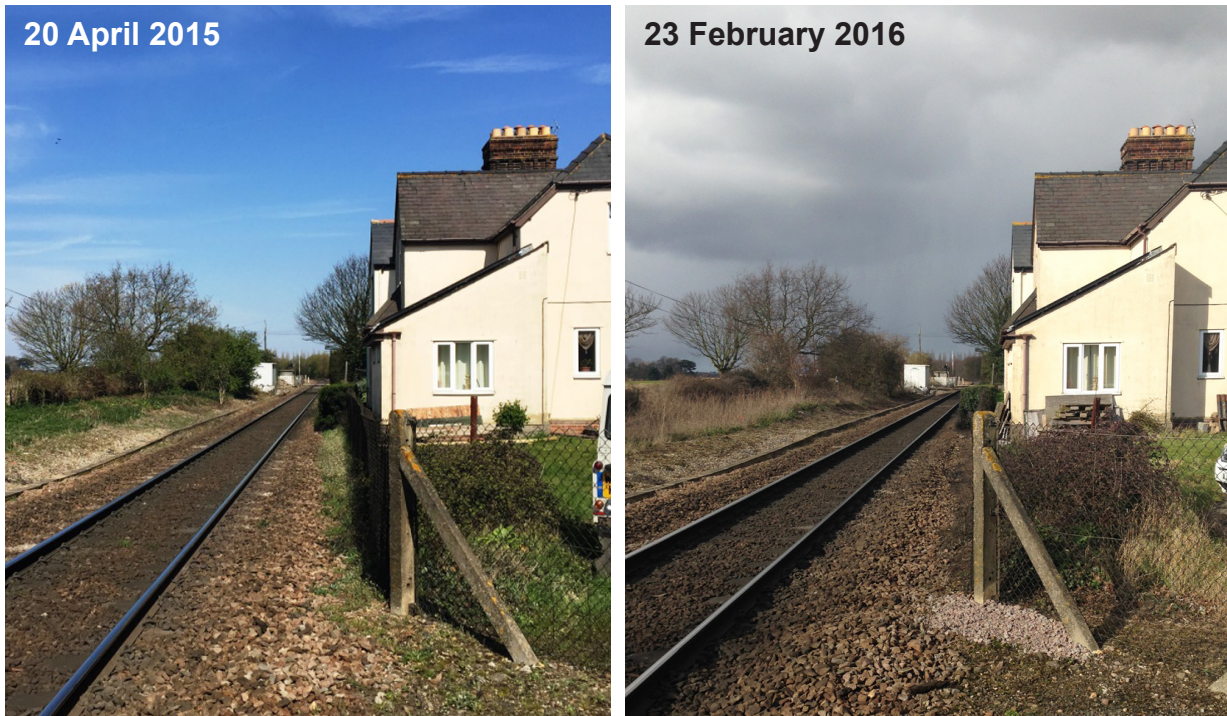
Figure 8: Photographs taken from the east side of the crossing, in the direction from which the train approached, on 20 April 2015, for the last level crossing risk assessment, and 23 February 2016, after the accident (images courtesy of Network Rail)
