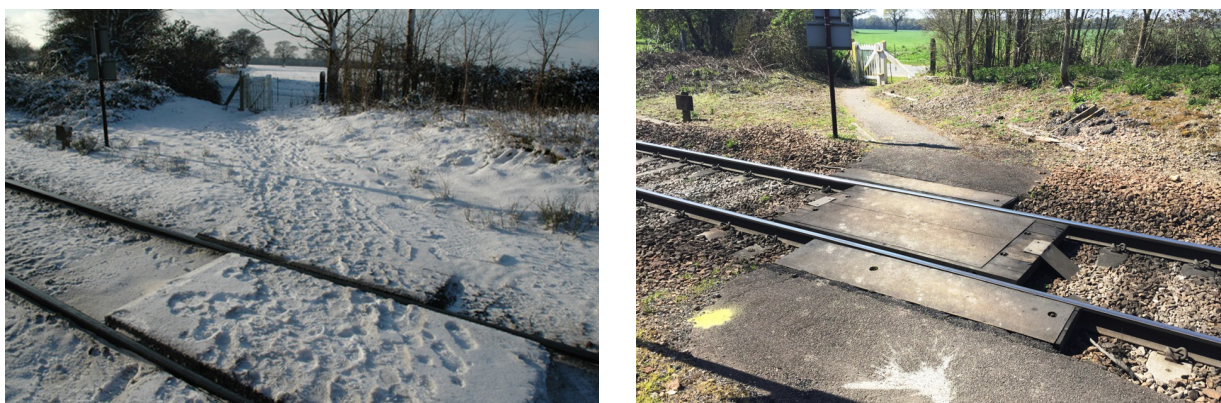
Figure 9: Evidence of footprints and wear marks on the crossing deck (images courtesy of Network Rail)
