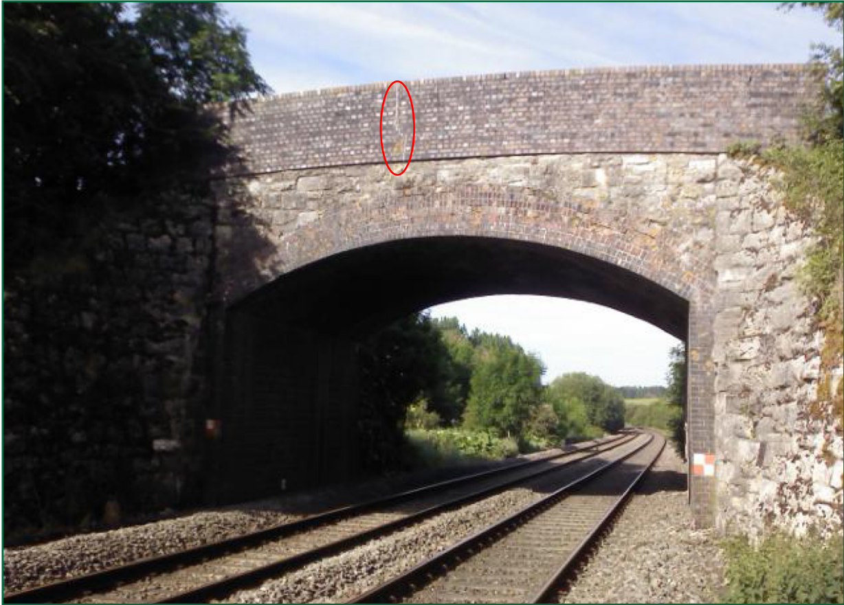
Figure 8: Crack in the eastern parapet (circled) as recorded in Network Rail's visual examination report of 12 June 2014
