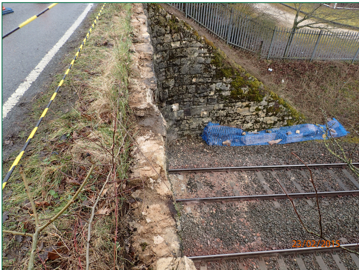
Figure 9: Location of failure of the parapet
