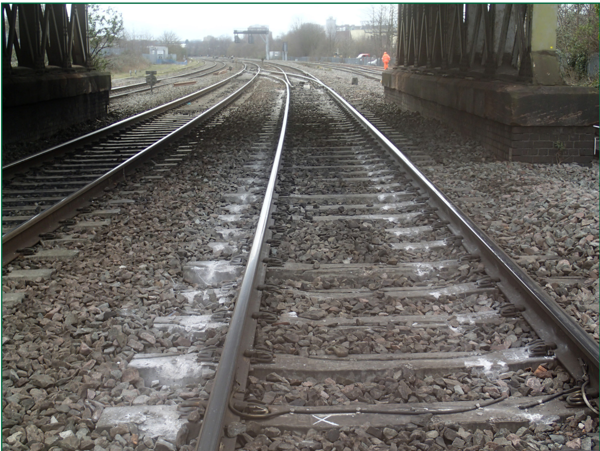
Figure 6: Damage caused to track by the derailed bogie
