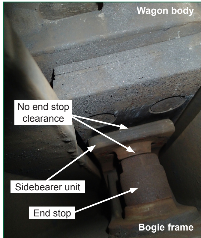
Figure 13: Sidebearer on the left side of the bogie which derailed, showing no clearance between sidebearer casting and end stop (arrowed)
