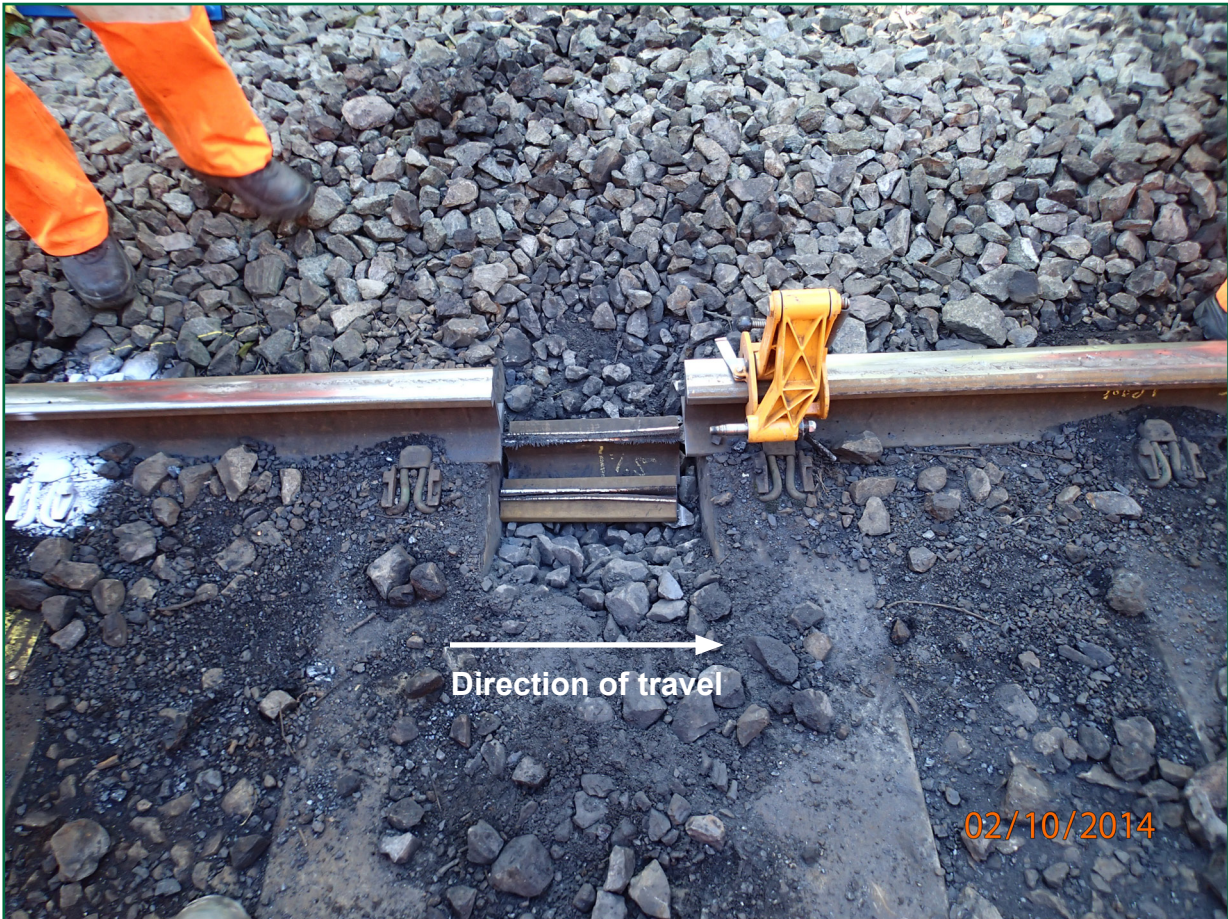
Figure 11: Apparently intact rail on the approach to the point of derailment
