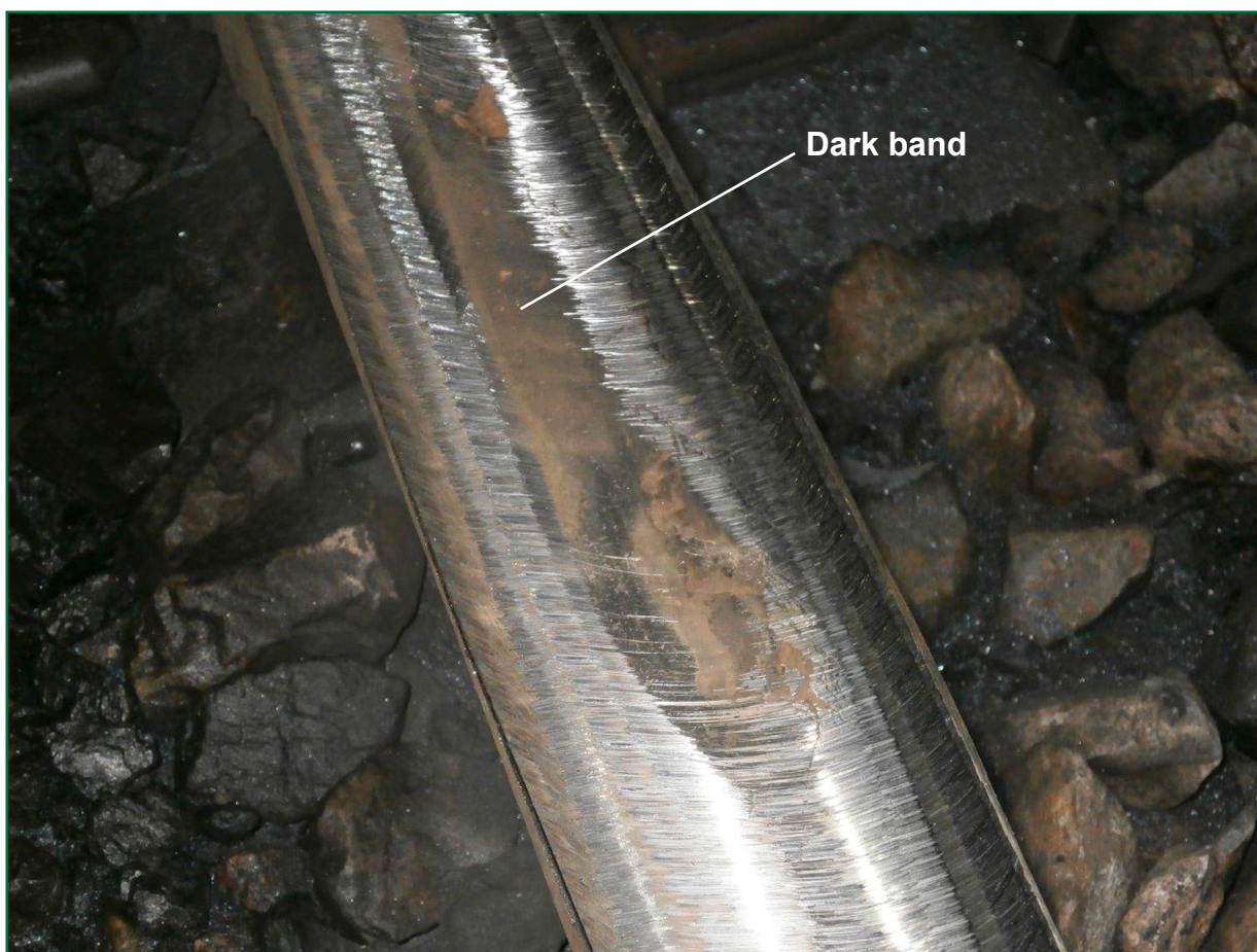
Figure 16: Photograph of left-hand rail taken by Harsco after grinding on 30 August 2014 (dark area shows where rail had started to collapse)
