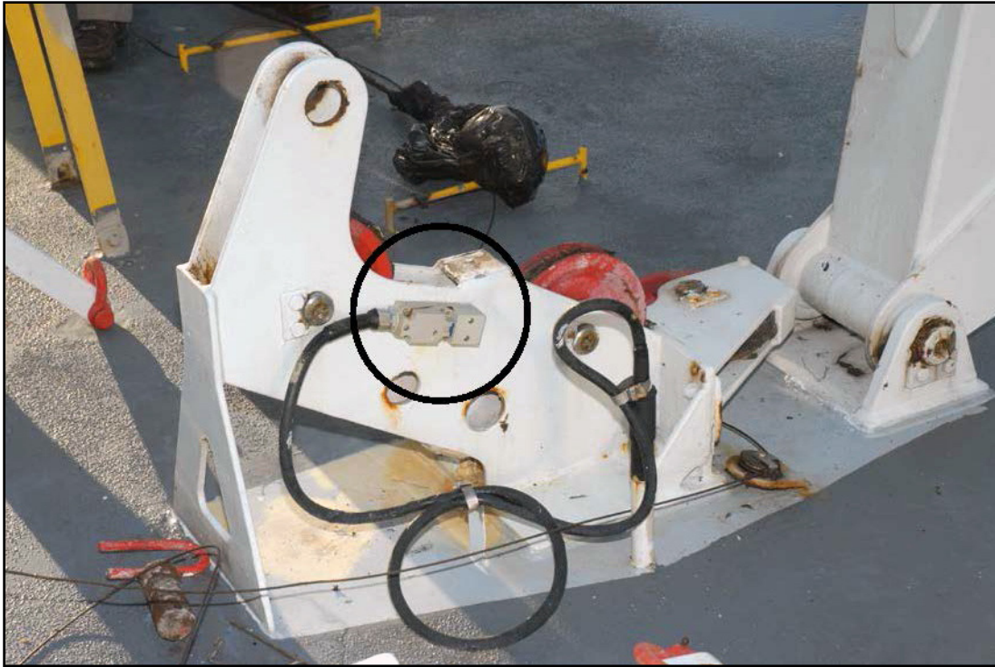
Figure 2: Proximity switch on davit (circled)
