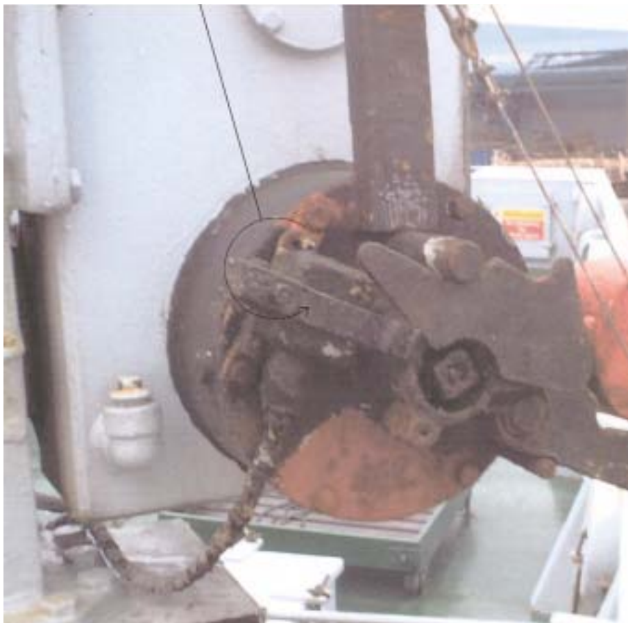
Incorrect position of interlock switch lever
