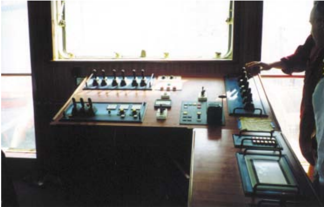
Winch control panel
