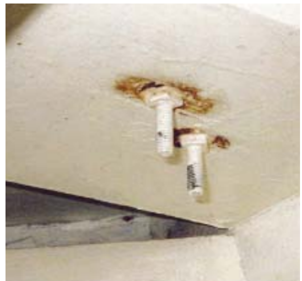
View from under sheared bolts before removal
