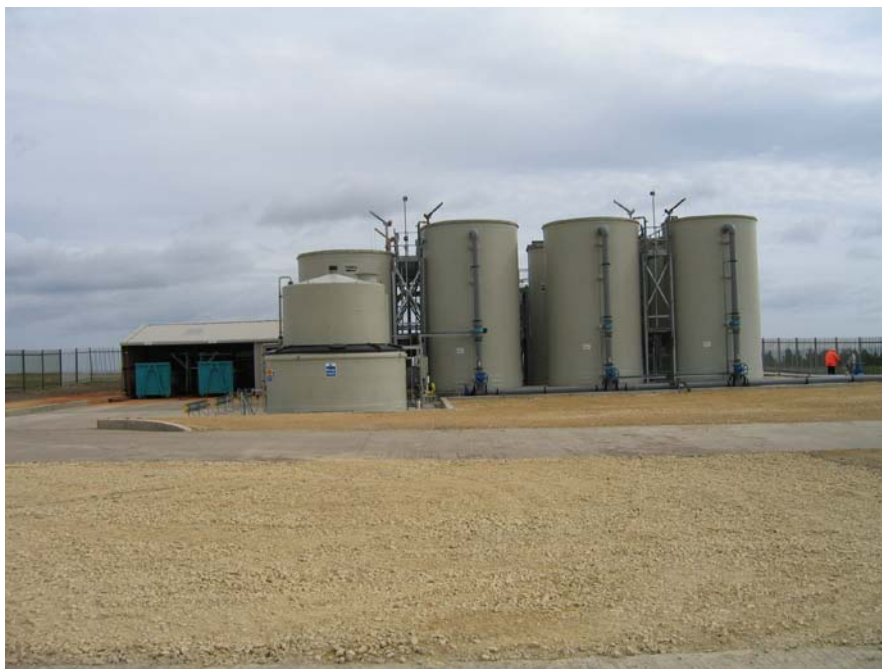
The Coal Authority Photograph – Active Mine Water Treatment Scheme Horden, Durham
