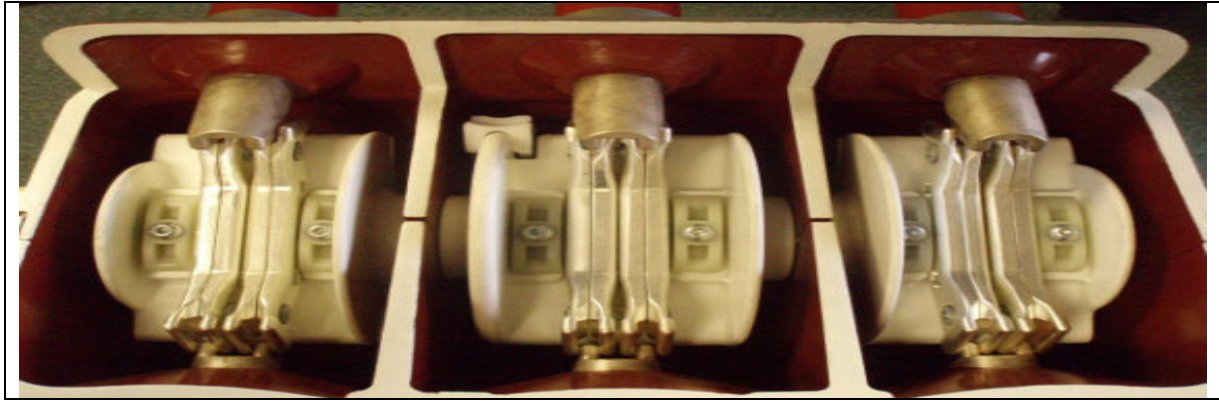
Figure 3: 1250A Disconnecter Contacts
