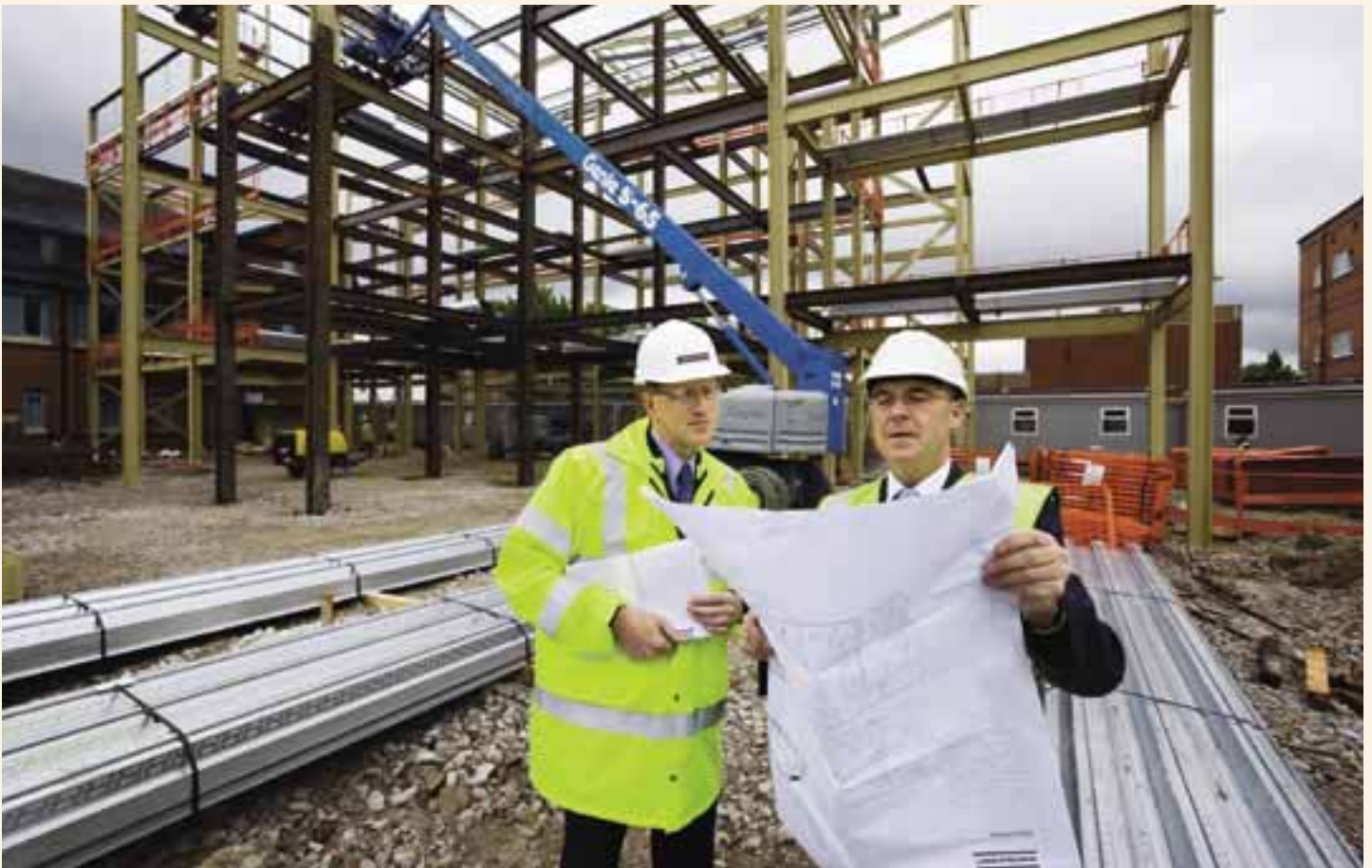
Dr Chris Burke (right) on site at the construction of the new Cardiology and Surgical Unit
