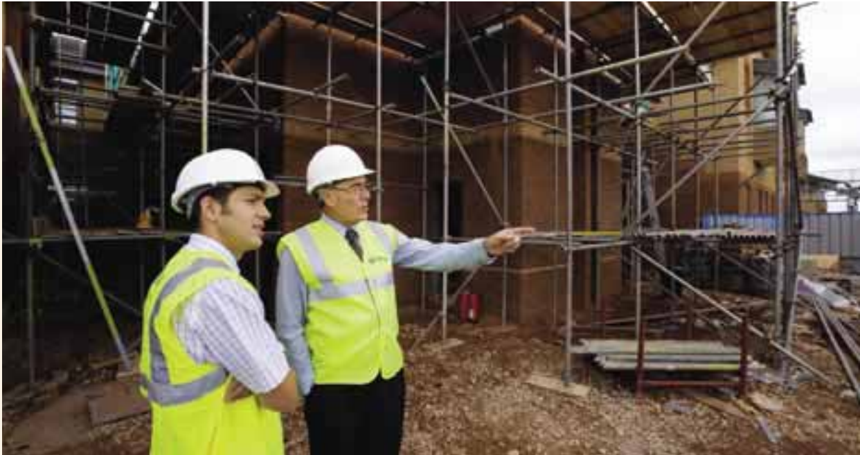
Above: Dr Vaughan Pierce, Medical Director (right), surveys the site of the new Cardiac Catheter Laboratory which is under construction
