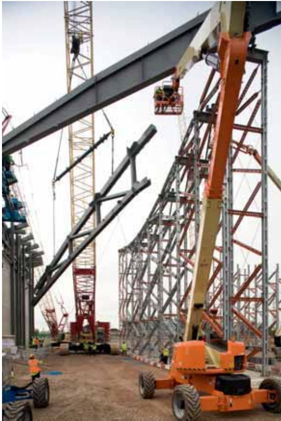
The Aquatics Centre - Progress - Roof steel lifted into place March 2009 Photo courtesy of London 2012
