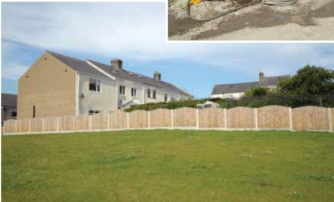
Subsidence damage repairs in the North East
