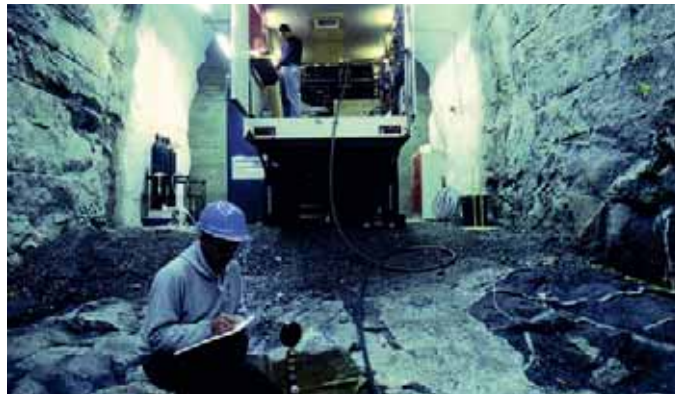
Part of a Geological disposal facility under construction in Finland (courtesy Posiva)
