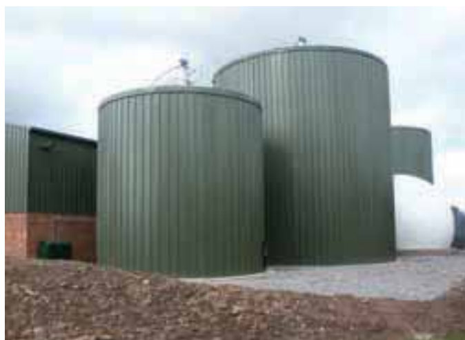
Greenfinch anaerobic digestion plant in Ludlow – renewable power from food and garden waste.
