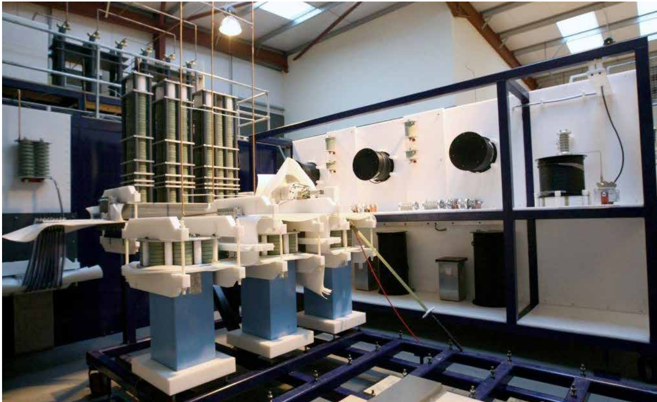
Cardiff University Morgan-Botti Lightning Laboratory, tests composite materials including those on the A350 XWB wing
